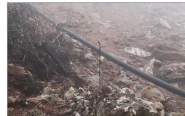
A landslide swept away the main water line for Namchi.
