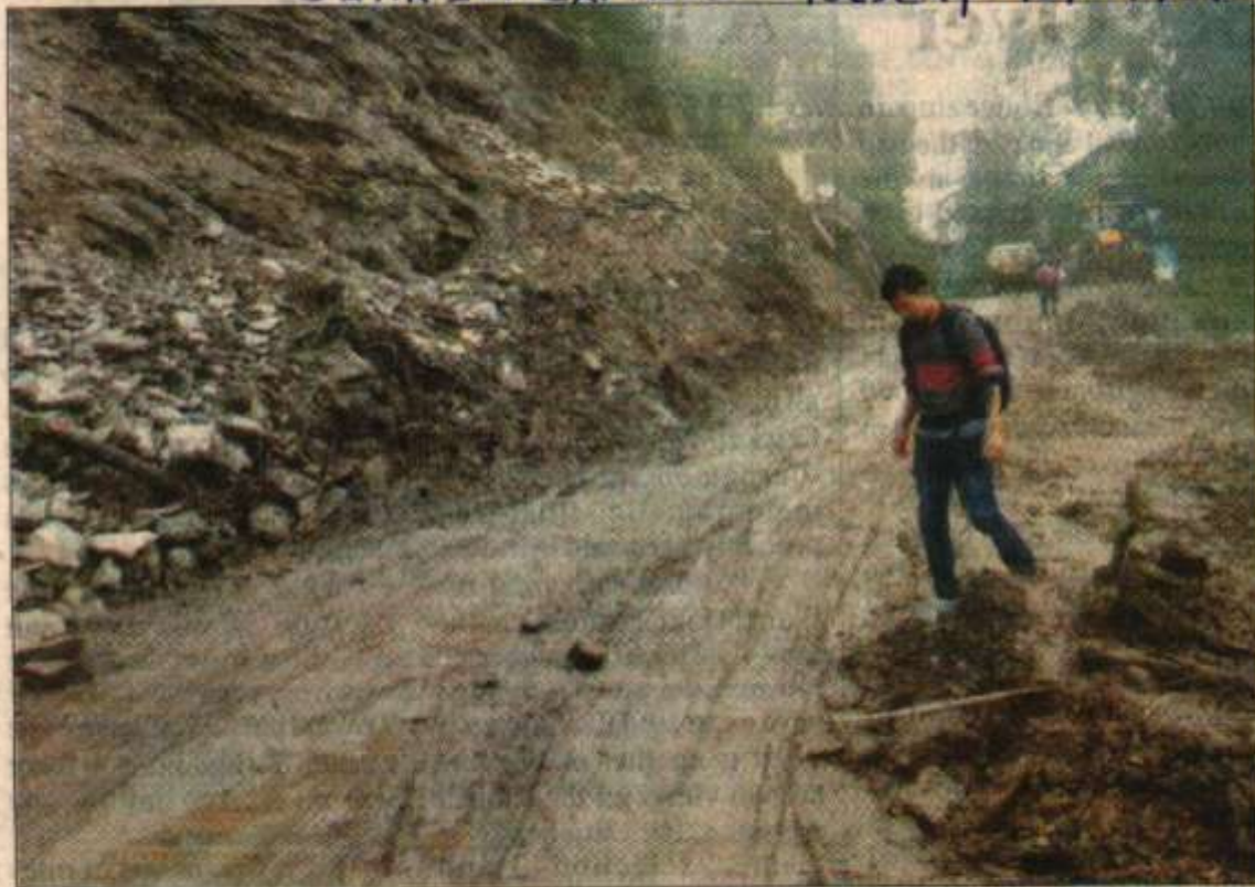
Traffic has been unpredictable on the Pakyong-Pachey SDM office road since Sunday. In less than 48 hours, the road was blocked on 3-4 occasions due to mudslides. An earthmover has been placed on the site for immediate restoration of road in case of any further landslides. (AJAY THAMI)
