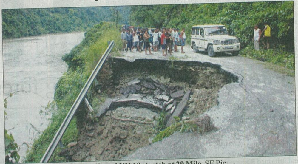
The affected NH 10 stretch at 29 Mile. SE Pic
